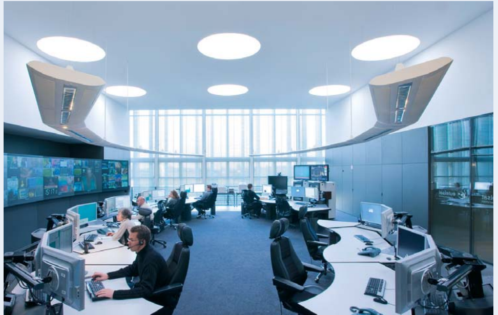
Eutelsat's communications system control centre at its Rambouillet teleport
